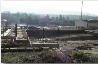
The Big Dig-Construction delays opening of Calaveras high school swimming pool.
